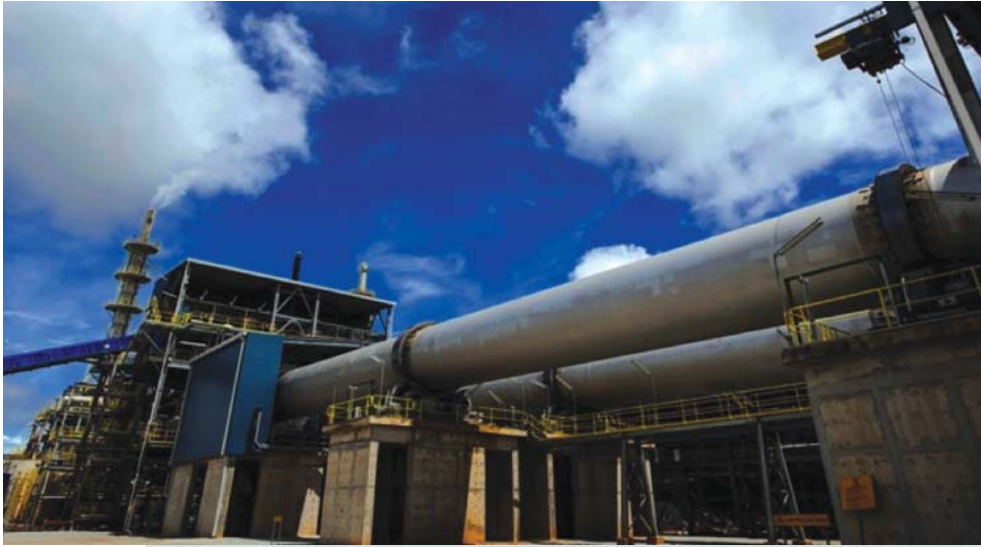
Two gas-fired kilns used to process REE concentrates at the Lynas Advanced Materials Plant, which has been intermittently closed as the new Malaysian government urges the company to solve what has been called a “radioactive waste” issue. (Image: Lynas Corp.)
